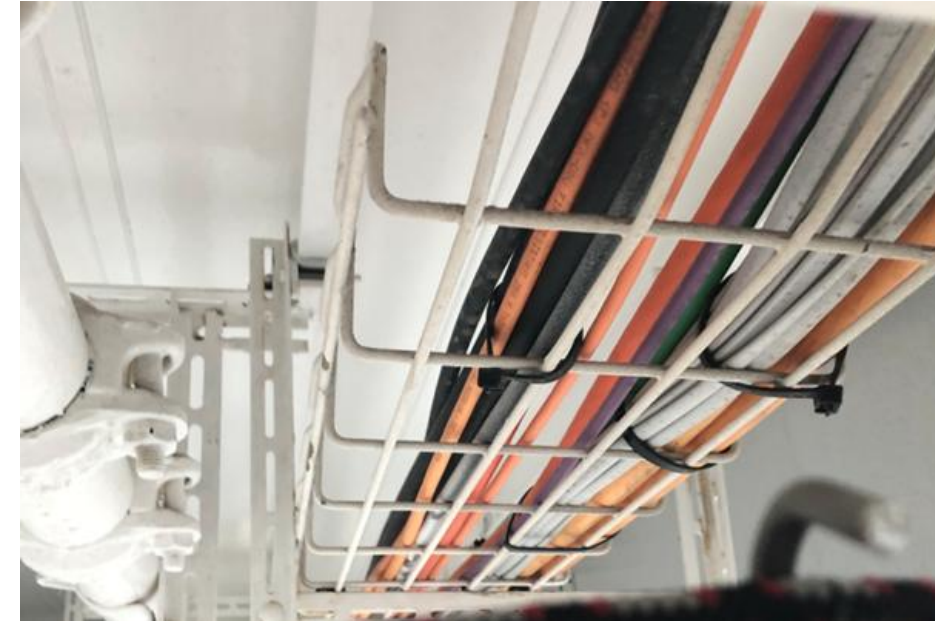
Cables on Emerald Princess (Photo by Norbert Doerry)
